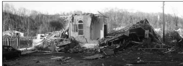
St. Luke's Catholic Church in Salyersville, Ky., suffered severe damage in a March 2 tornado. PHOTO CONTRIBUTED BY CAMPUS MINISTRY
